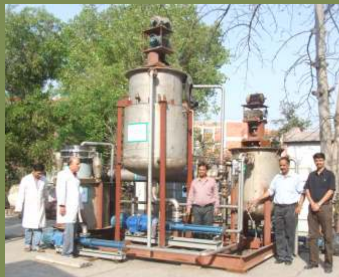
Commissioning of Pilot Plant for Removal of Non Process Elements at CPPRI
